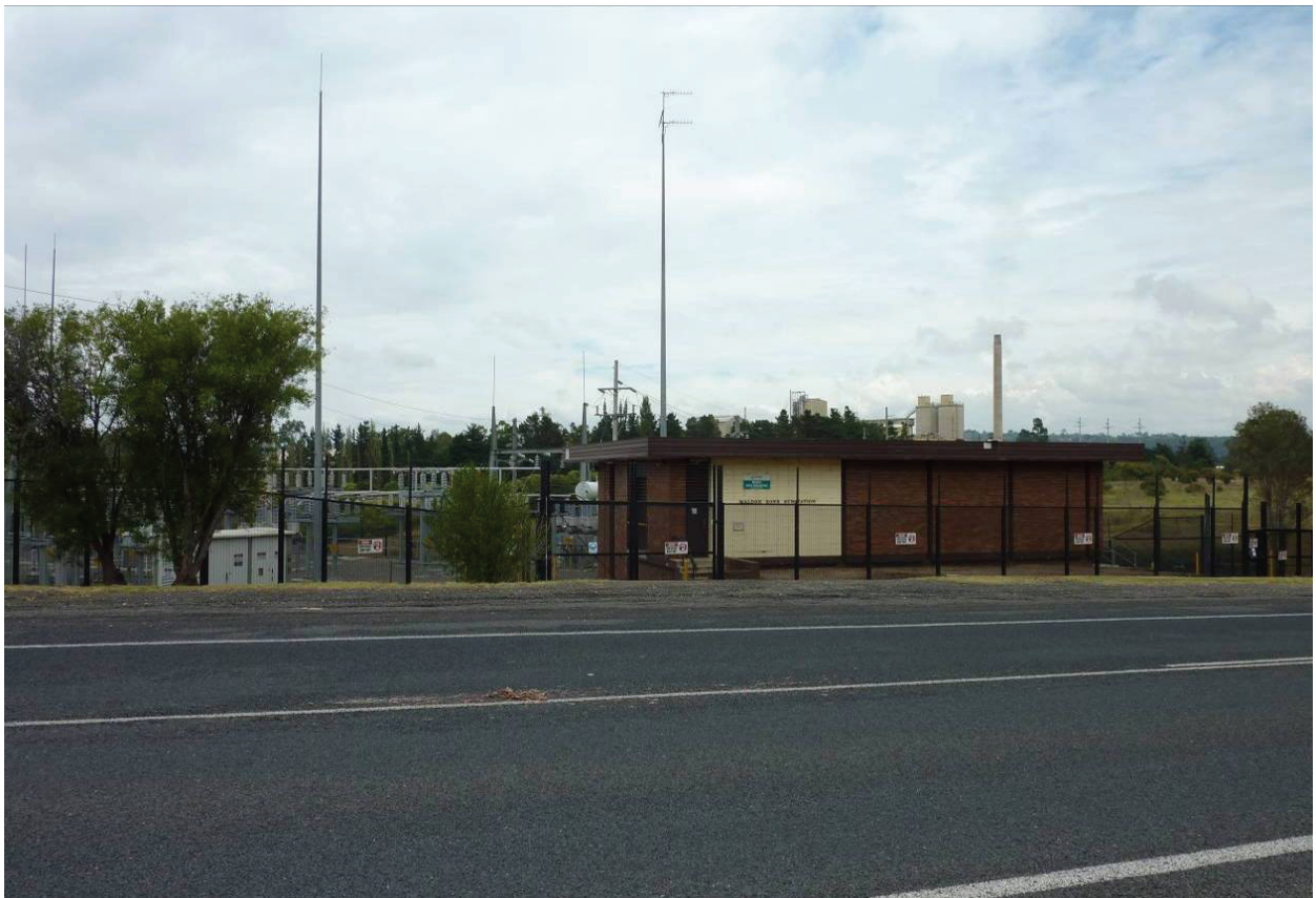
Plate 5.6 Maldon Zone Substation
